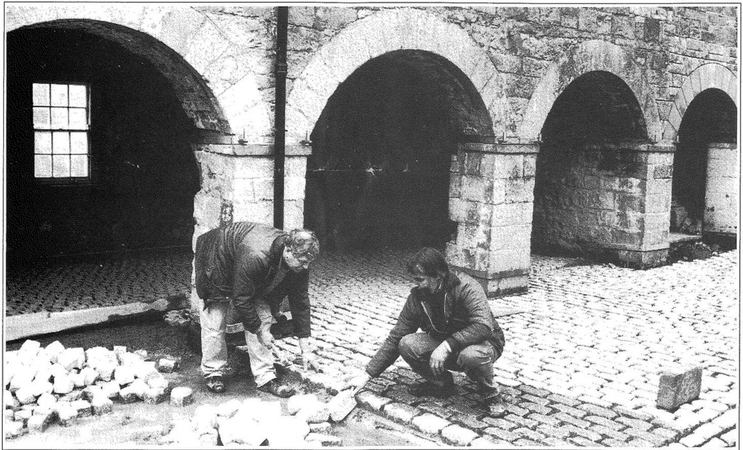
William McFrederick and Reggie Dixon of the Environment Service laying setts in the arcaded range of the Castle Barracks yard.
