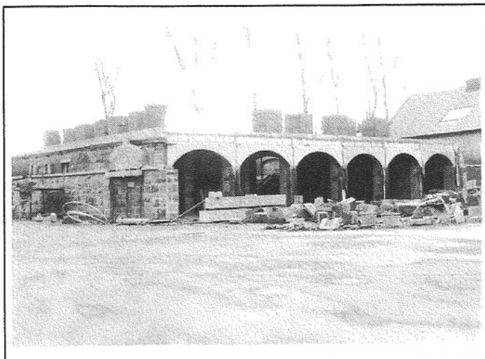
Work in progress in the new Heritage Centre in the Castle Barracks, Enniskillen.
